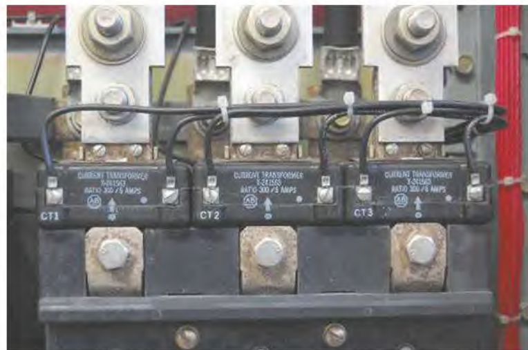
Figure 4-33 Large starters are often provided with current transformers.
